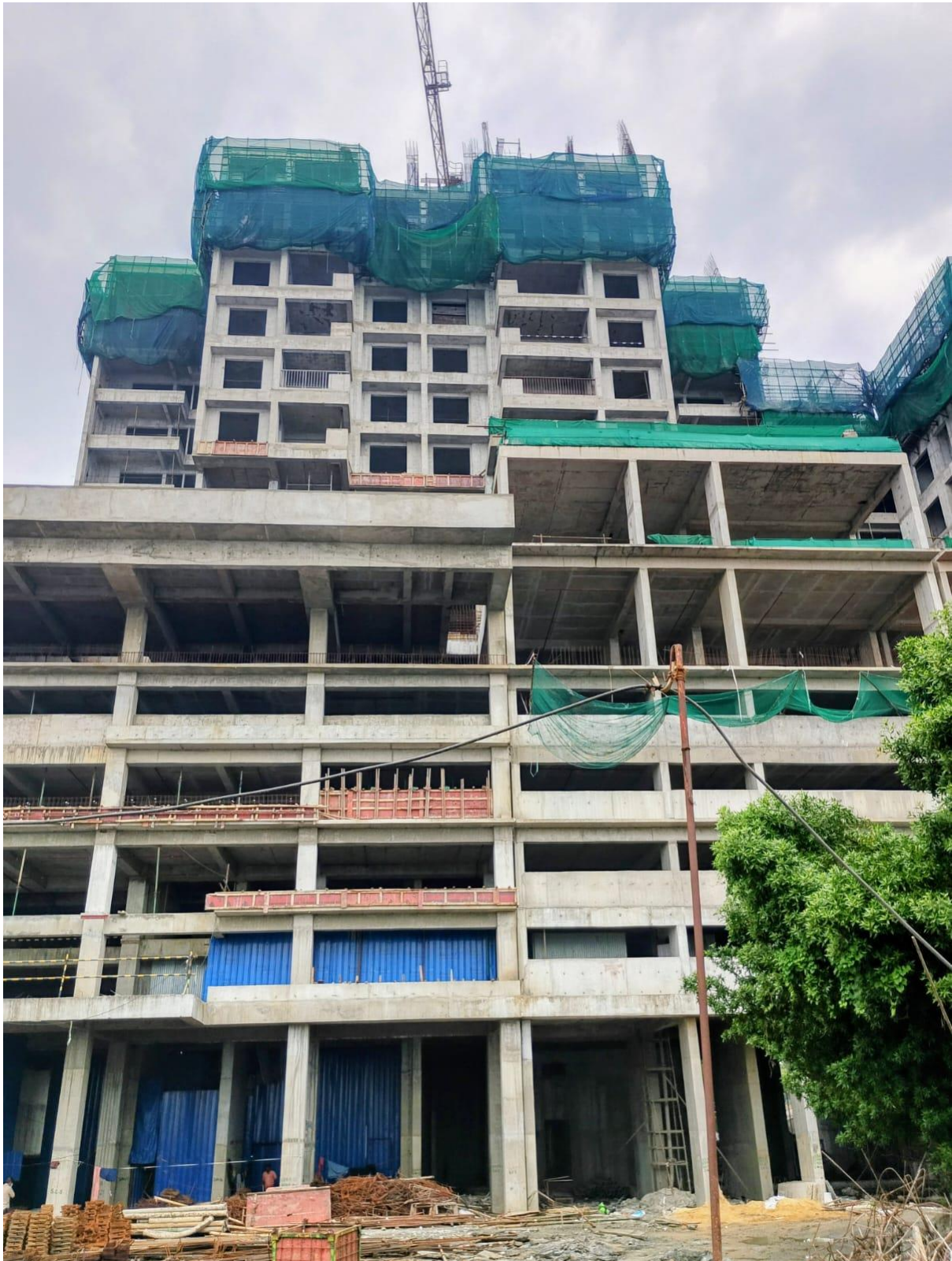
Tower 13 – Super-structure work in progress i.e. 15 th slab work in progress & swimming pool work in progress.
